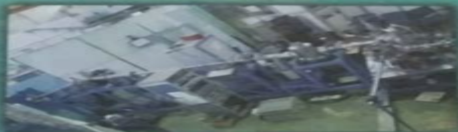
Photograph of a large industrial facility, likely a power plant or refinery.
